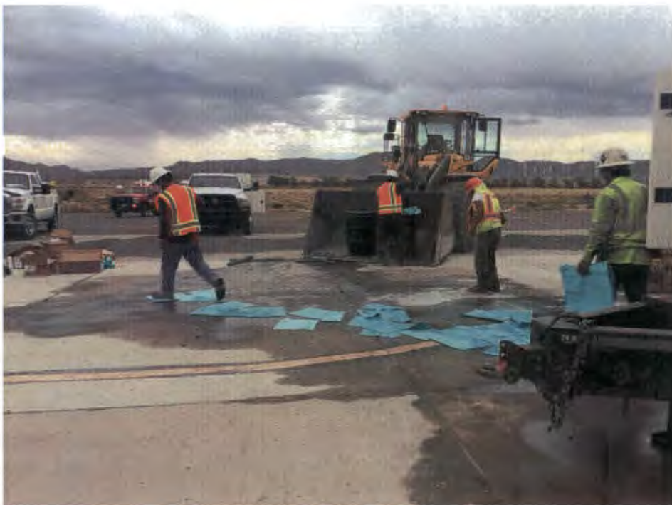
Spill looking west from generator
