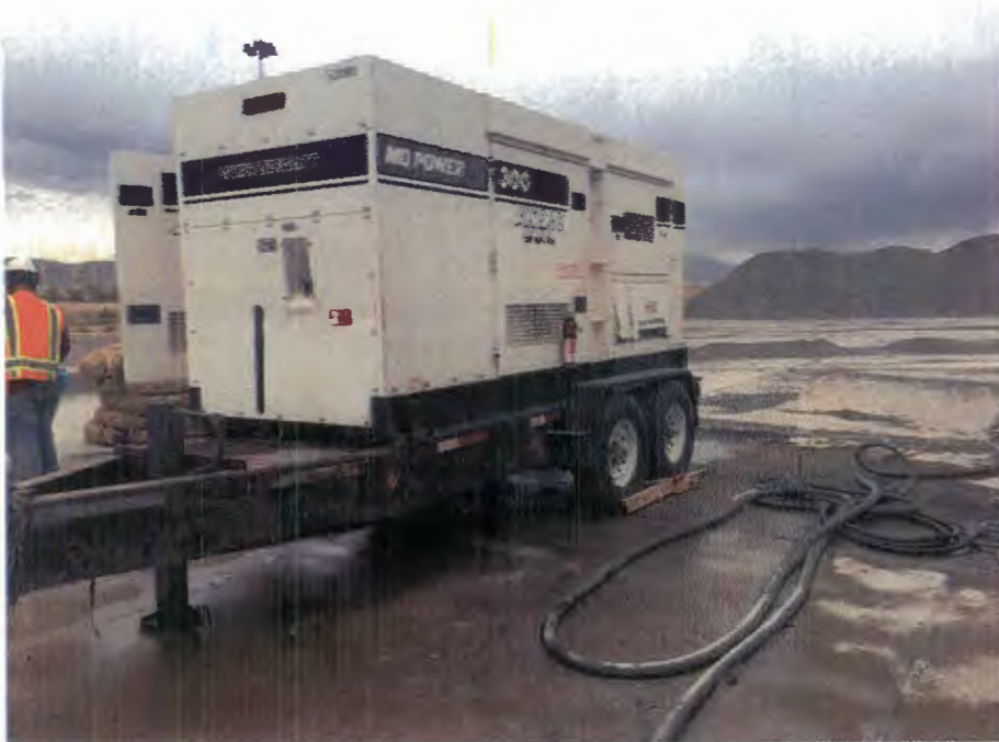
Portable diesel generator
