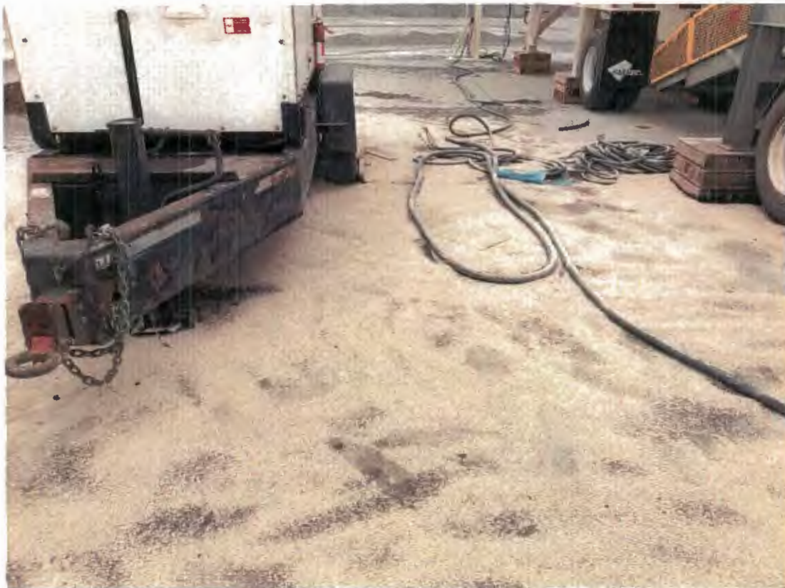
Spill cleanup in progress
