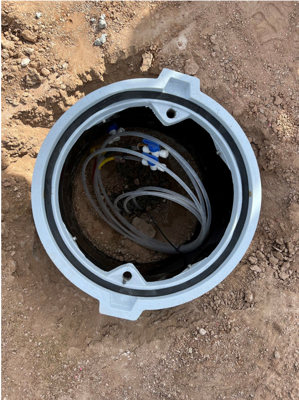
Figure 5-6: Well Vault and Vapor Probes Photo
