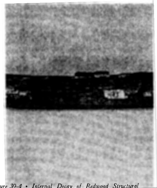
Figure 39-4 • Internal Decay of Redwood Structural Member Showing White Fungus Mycelium
