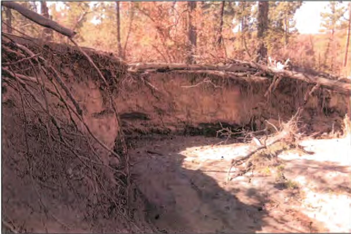
Photograph 3. Severe bank undercutting.
