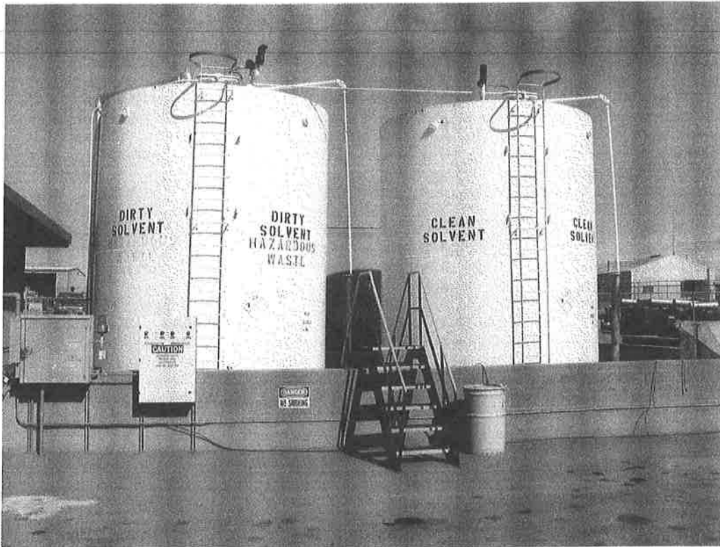
Photo 1: Secondary Containment Area and Tank System
