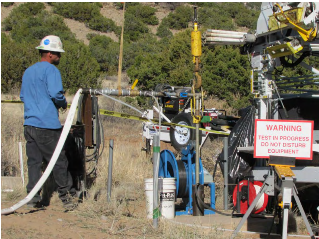
View to the North. Pump Puller Rig (right) and Discharge Line Setup in the Burn Site Well.
