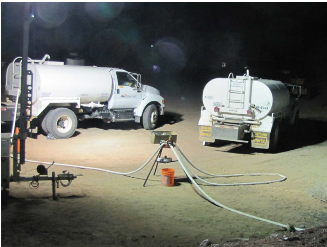
View to the West. System for Management of Groundwater Discharge, Lay Flat Hose from Burn Site Well (right), Splitter Valves/Hoses (Center), and 3,000-gallon Water Trucks (background).
