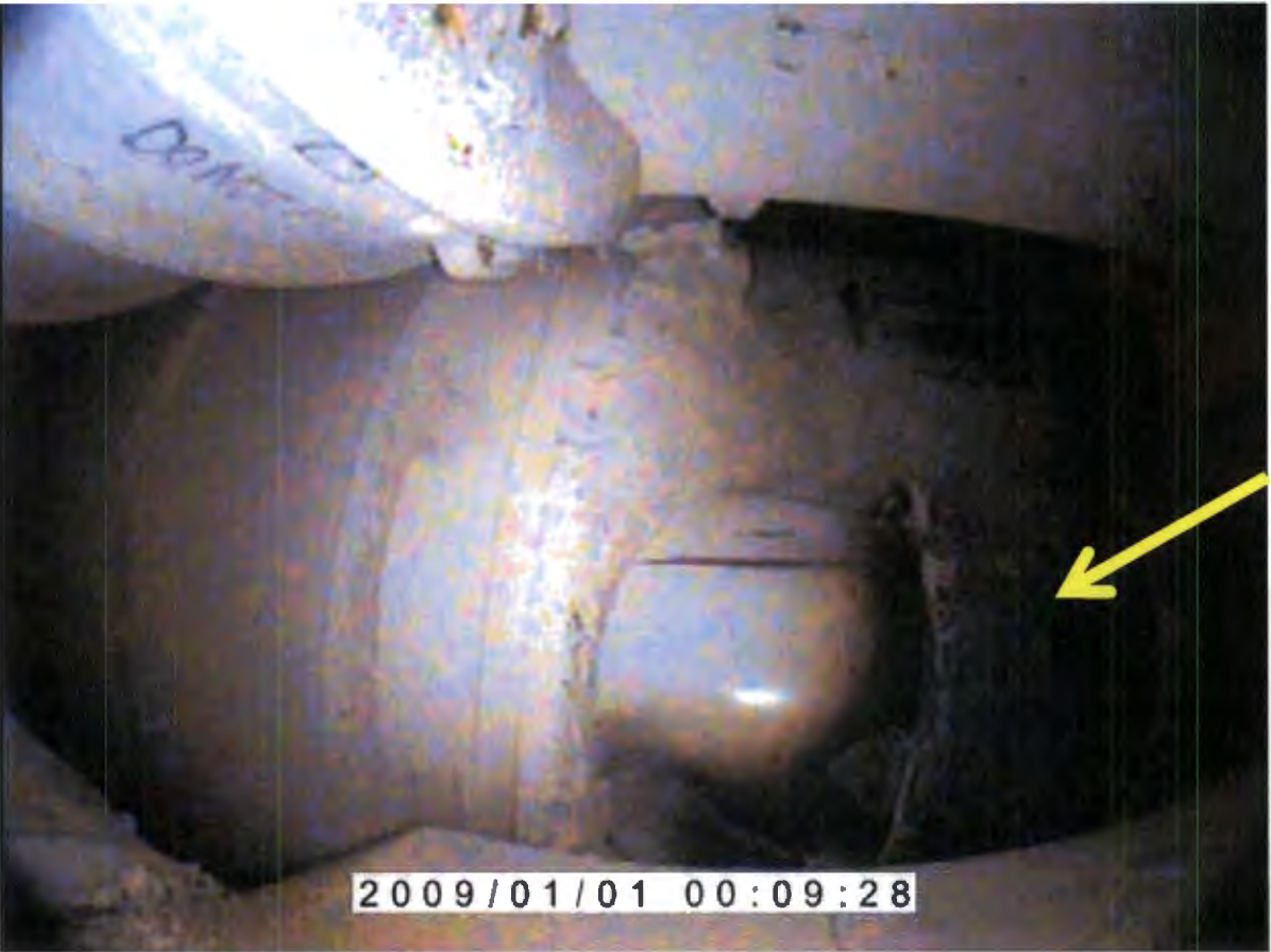
Drum that had lid breached
