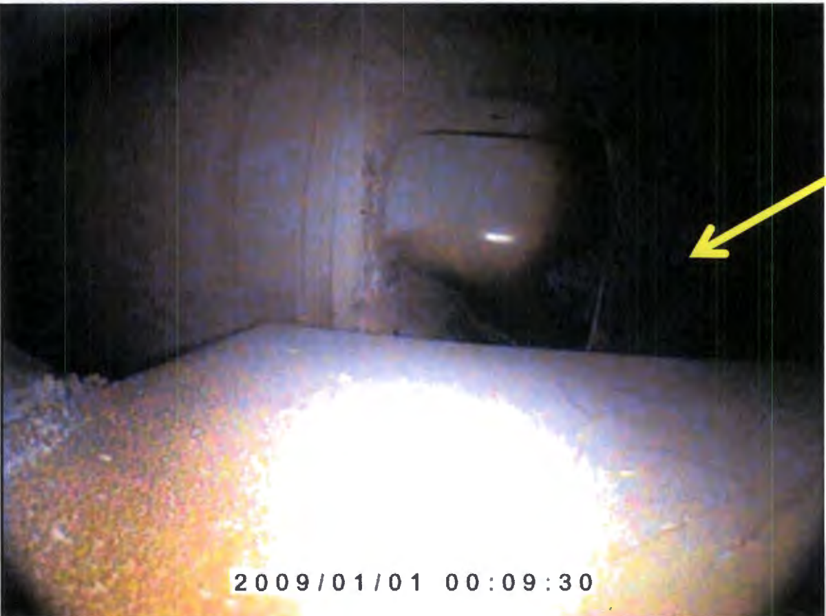
Drum that had lid breached
