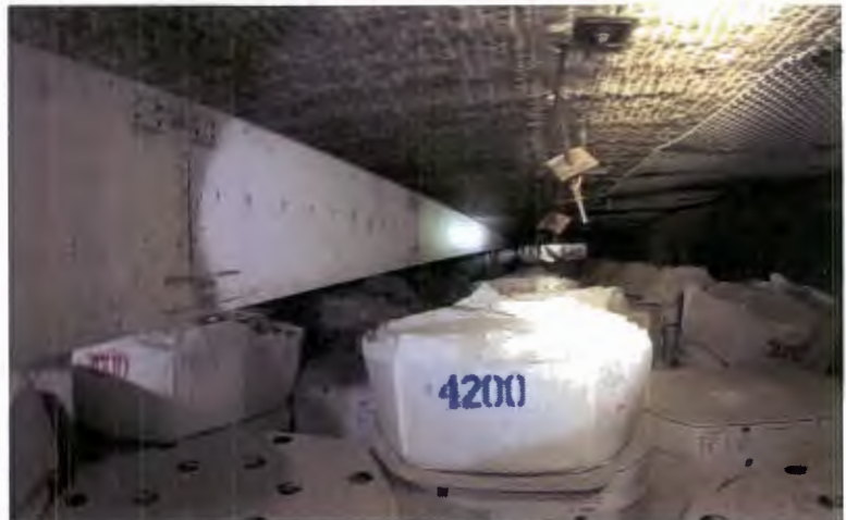
Project Reach's 90-foot boom is positioned over the top of waste containers in Panel 7, Room 7, as a remotely operated video camera collects photographic evidence.
