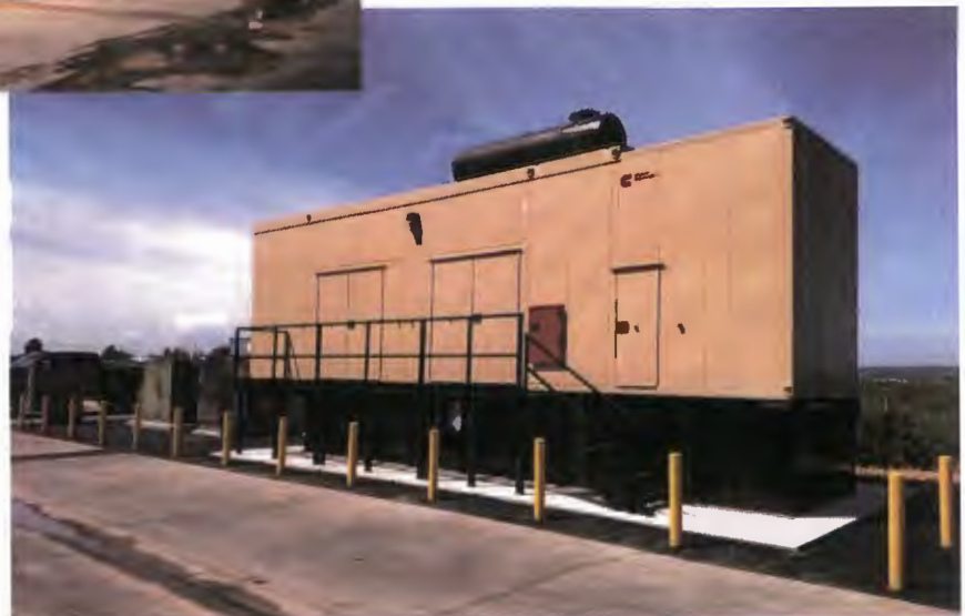
EOC Generator – Operational Ready
