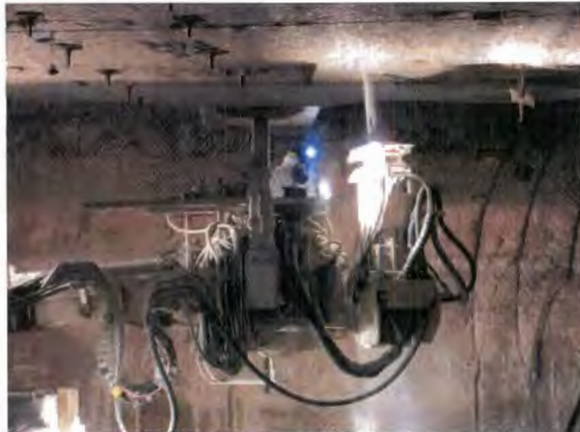
An Underground Operations employee, wearing anti-contamination clothing and a respirator, installs bolts in Panel 7 of the WIPP underground.
