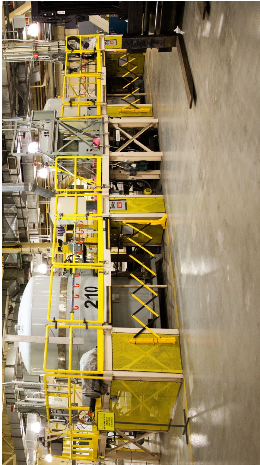
Figure B4-4 TRUDOCK (East) in CH Bay of the Waste Handling Building
