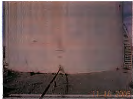
Close-up of old design tank on ground w/o secondary containment
