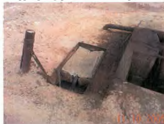
Chopper pump problem at API separator
