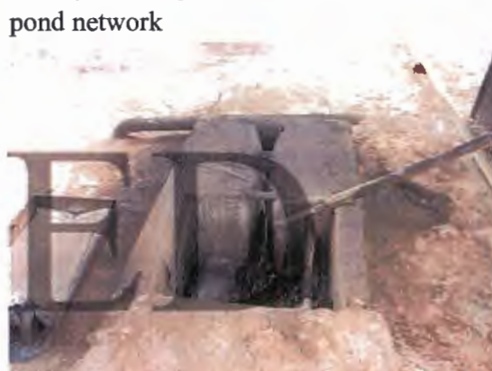
Chopper pump problem at API separator
