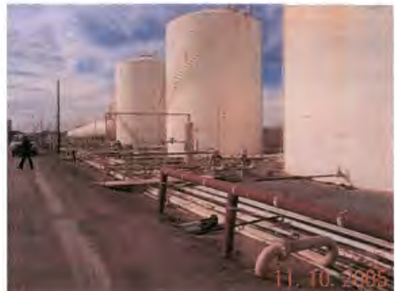
Looking S along pipe-rack on NW area of facility near Railroad Lagoon Rack
