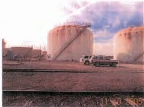
Tanks need berming at the NE area of the facility
