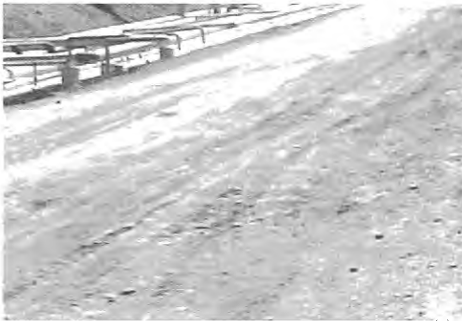
Figure 6: Preliminary clean-up of road which had experienced run-off of product.
