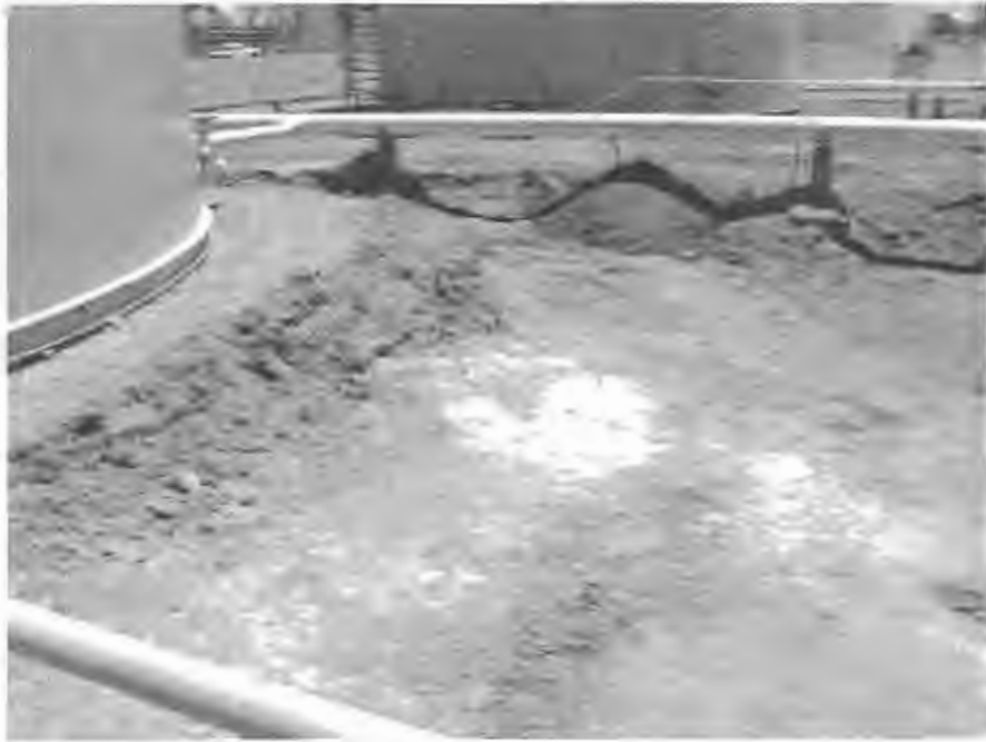
Figure 4: Excavation of contaminated soil in the area described in Figure 2. Note active pipeline towards the rear.
