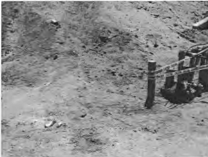
Figure 5: Preliminary excavation of contaminated soils near the drain pipes where product flowed out from the open foam line within the tank
