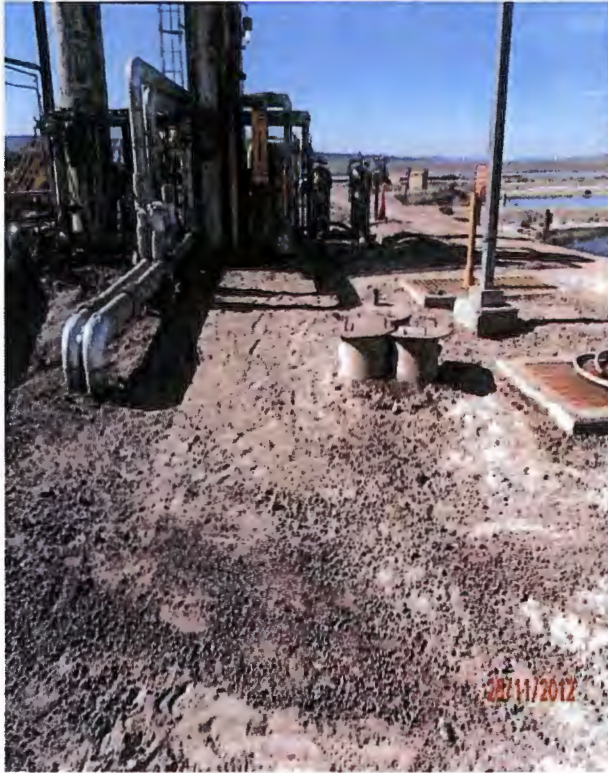
East side of the benzene strippers
